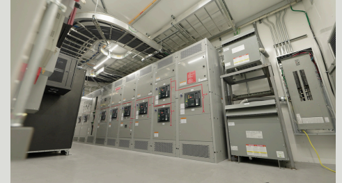
Power Distribution Center
