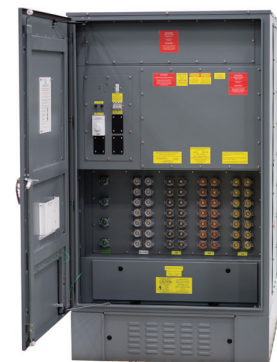
Generator Docking Stations
