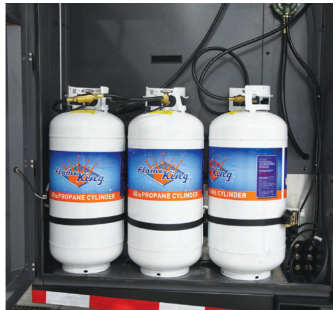
LP Tank Storage Cabinet Interior
