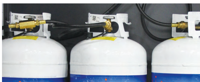
Tank 3 Extreme Left
