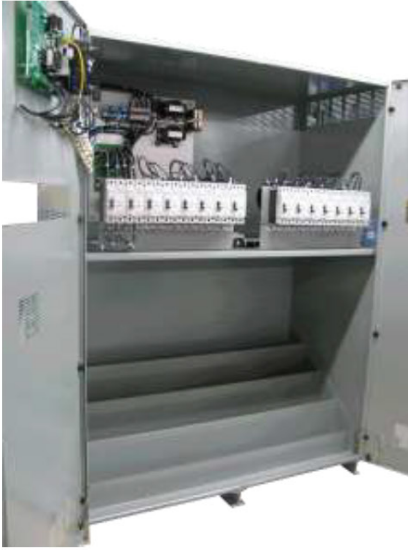
Charger with integrated DC distribution panel and battery compartment
